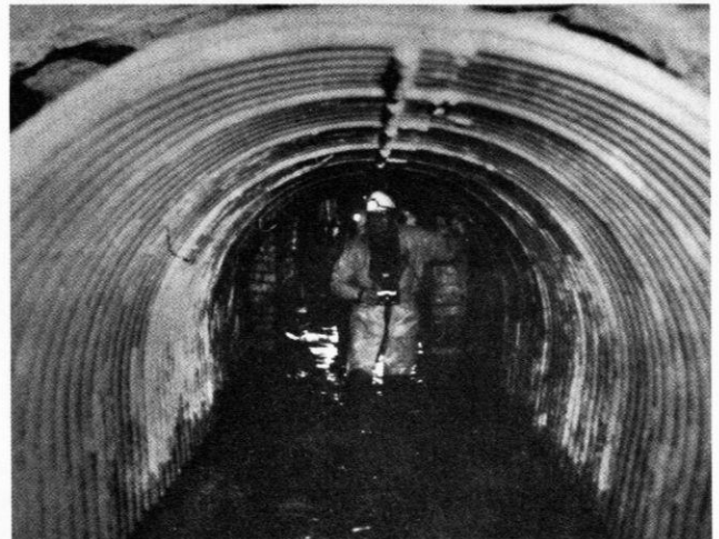
Sub Brit's former secretary Malcolm Tadd in the lined section of tunnel near the entrance - Photo by Michael Jack
